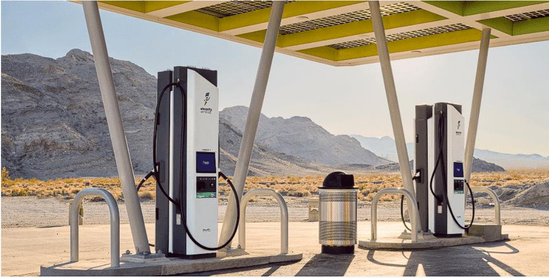
Electrify America EV Charging Station
